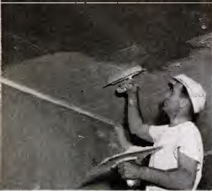
Photo above shows base coat of lightweight-aggregate plaster being applied. Ready-mixed avoids common problems of using bad sand or oversanding
